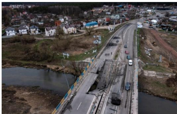
Fig. 1. A partial collapse and craters in the deformed superstructure reduce the load-bearing capacity of the structure. How reliable is the bridge?
