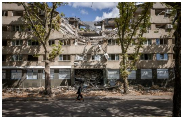
Fig. 2. The damage to the building is considerable. Under what conditions can it be used safely and for what purposes?
